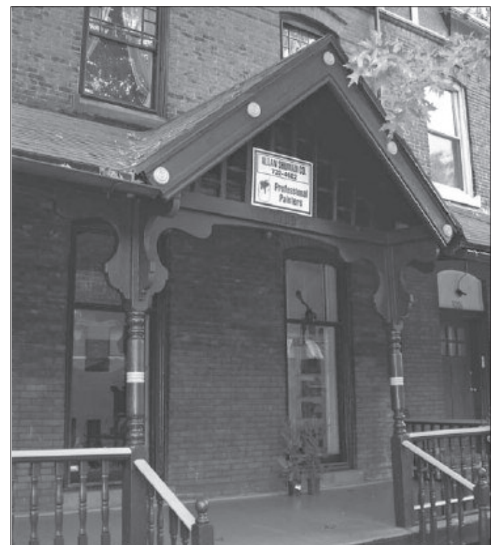
1008 South 49th Street is a Queen-Anne style twin house in West Philadelphia; restoration included the repair of eaves and gutters, stucco, woodwork, and painting the exterior in a three-color Victorian palette.
