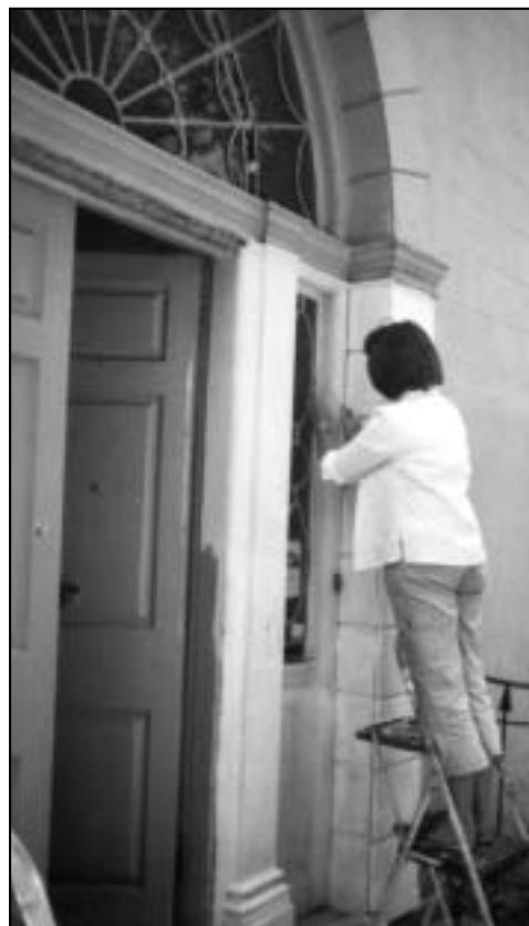
Conservator removes deteriorated finishes from the main entry of Lemon Hill, a project funded by the William Penn Foundation, the Friends of Lemon Hill, and the Fairmount Park Conservancy Historic Properties Fund.
